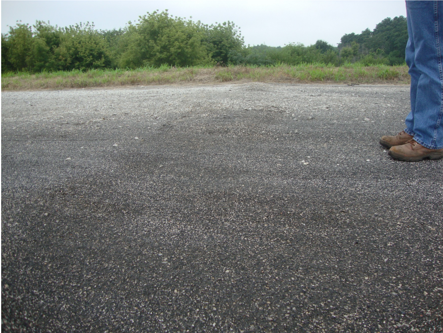
Compression heaving in crest of embankment
