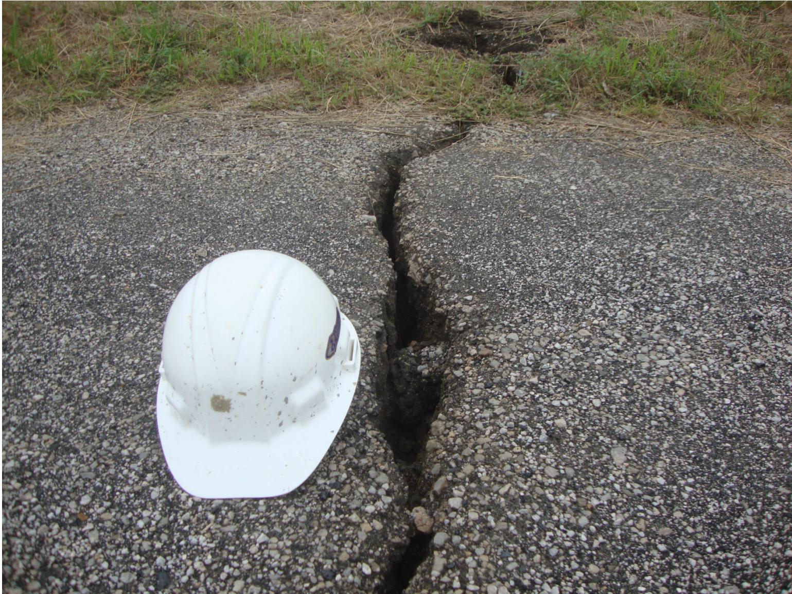
Tension cracking in embankment crest
