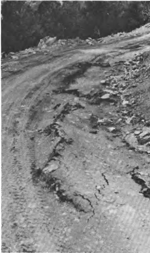
FIGURE 2.—Compression ridges produced contemporaneously with longwall mining near Raton, New Mexico.
