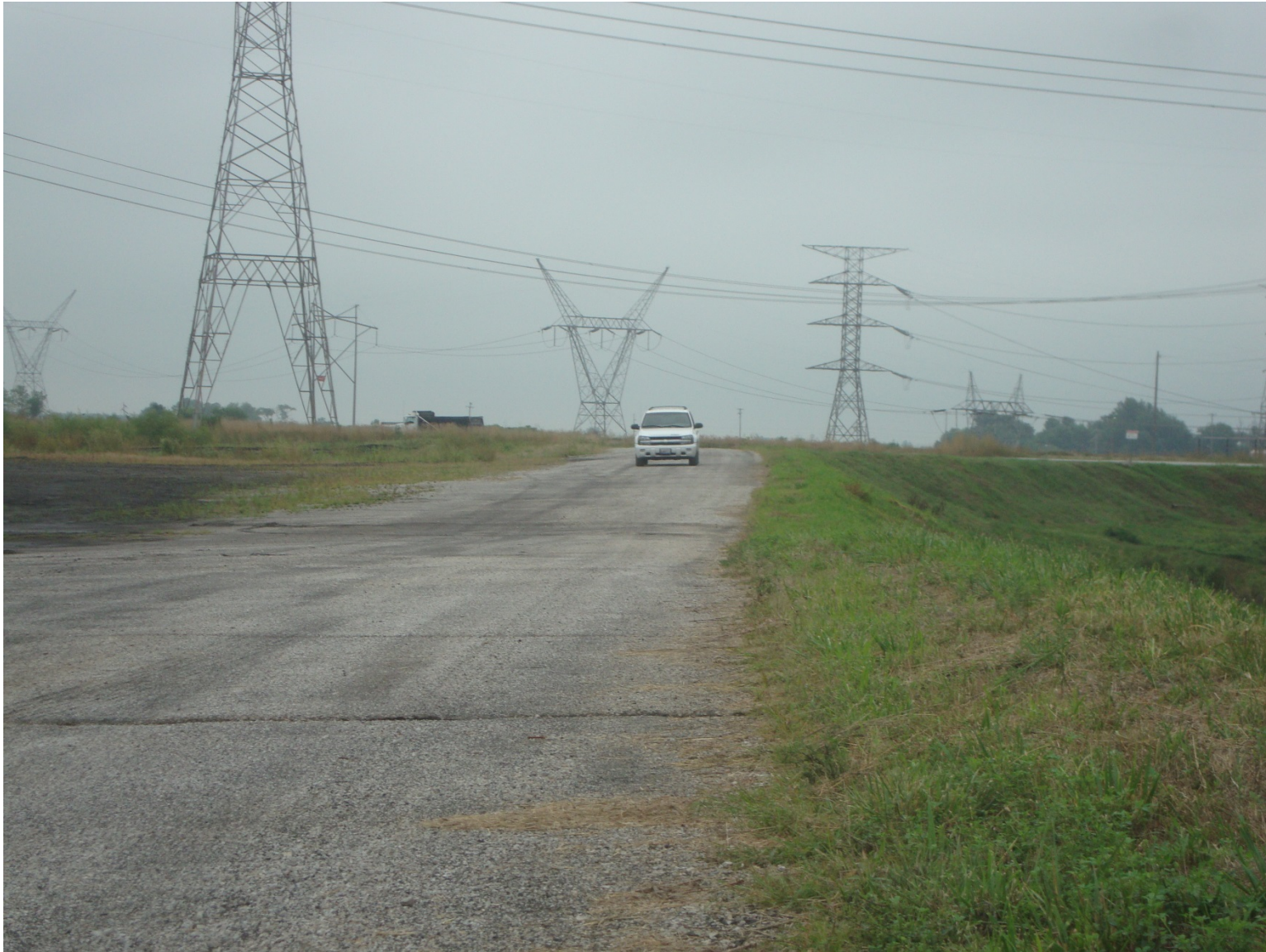
Depression in embankment crest and downstream slope, tension cracks visible
