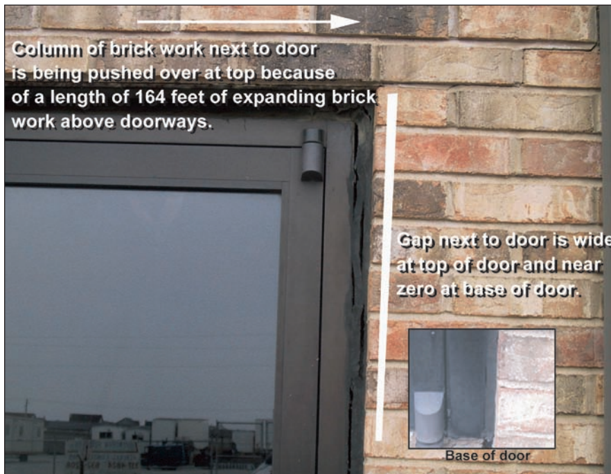
Figure 27 The long continuous length of brickwork above the door is expanding, pushing the top of the door frame to the right while the base of the door remains stationary. This movement creates the gap and causes the door to stick while opening and closing.
