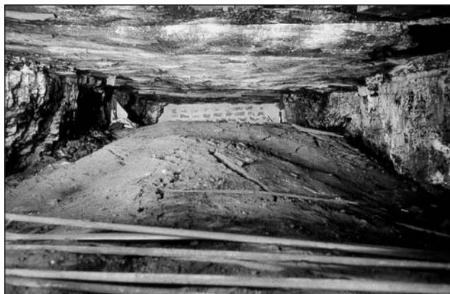
Figure 12 Diagram and photographs of coal pillars being pushed into a soft floor. The claystone material is being squeezed out from under the pillar up into the entryway.
