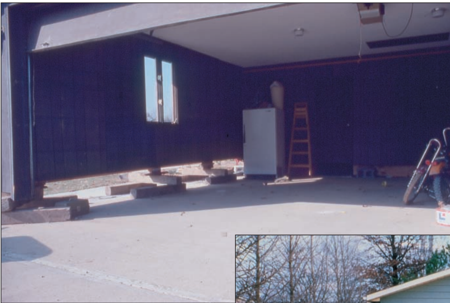
Figure 16 Load-bearing walls of a garage on a slab. The entire superstructure (frame) has been raised to a level position, exposing the interior of the garage. This re-leveling eliminates damaging stresses from differential movements of the foundation and maintains the superstructure level throughout the life of the event.
