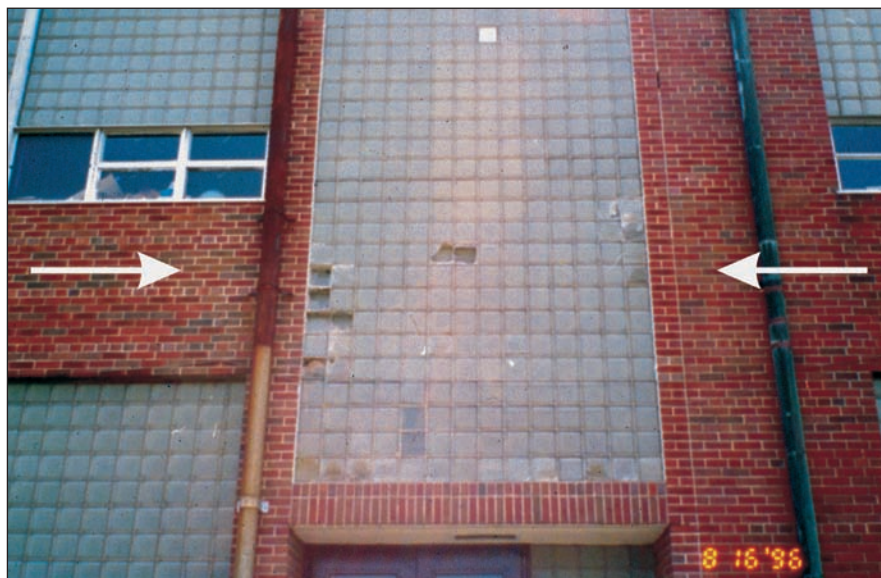
Figure 29 The long, continuous brickwork intersects the vertical glass block wall. Pressures have broken the glass blocks in line with the long continuous expanse of brick work.
