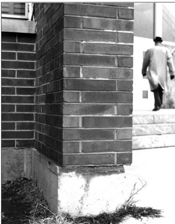
Figure 28 The largest movements are at the edges of the long continuous wall. At this point, the brick wall is being pushed off the foundation.
